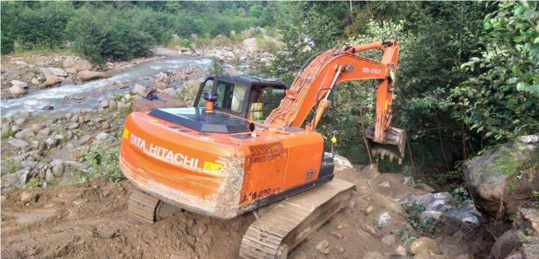
Fig: Track opening on Right Bank
